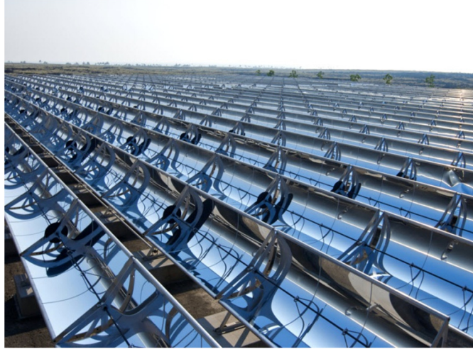
Figure 1-3 Parabolic trough solar collectors [6]
